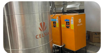
Thermal energy decarbonization project - Fund. Cardioinfantil
